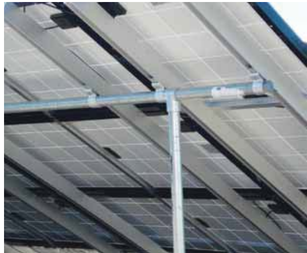
Check under the array for loose wires.
