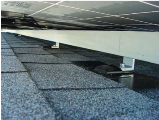
Check under the array for dangling wires
