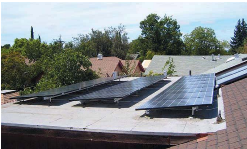
PV modules installed at shallow angle
