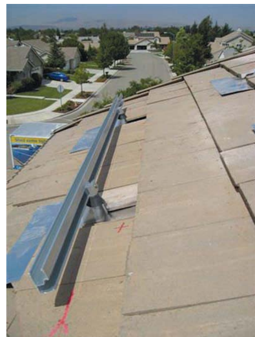
Down slope mounted rail
