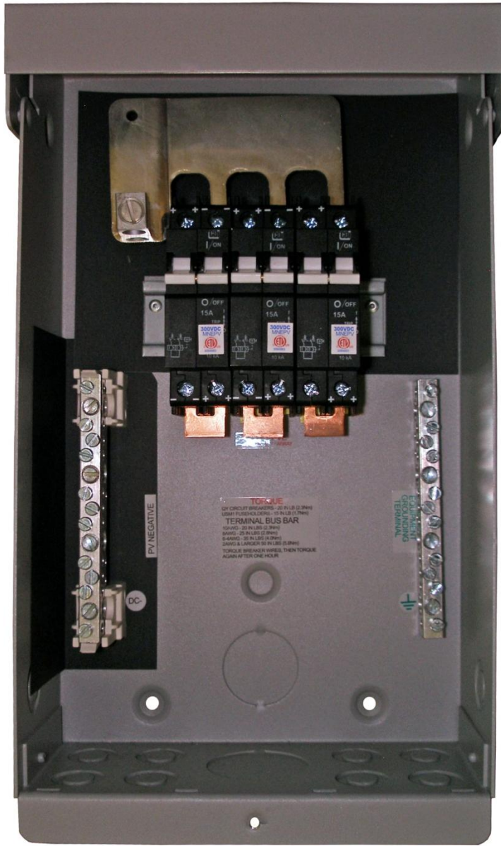
MNPV6-250 With (3) 300VDC Breakers installed
