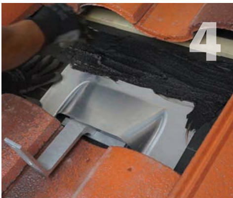
Apply 1/8" thick layer of roofing cement around the top and sides of the sub-flashing with at least 1" extending past the sides of the flashing onto the felt.
