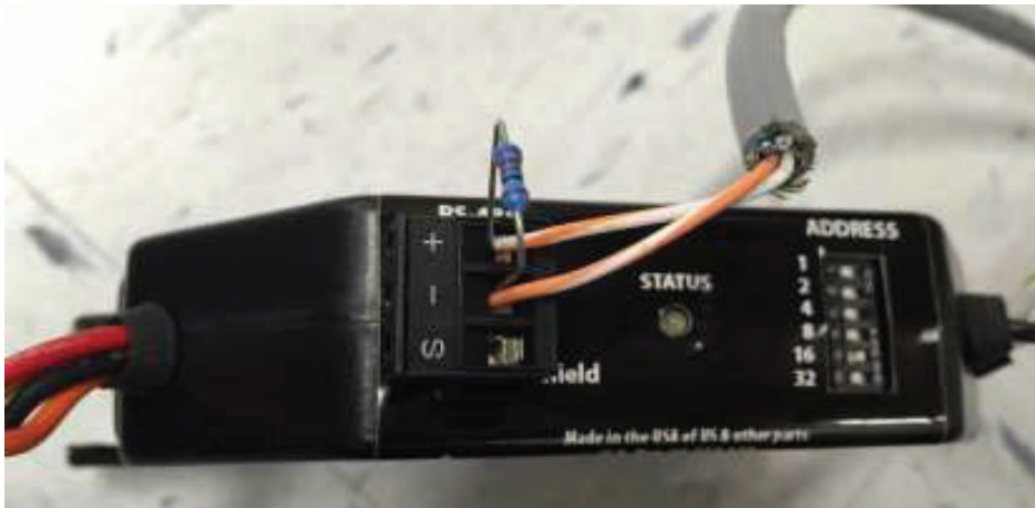
Figure 2.34 - This figure shows how the Veris RGM meter is connected to the Modbus (RS-485). Note the 120 ohm Modbus termination resistor (not supplied) is only needed if the RGM is the last device in Modbus daisy chain.
