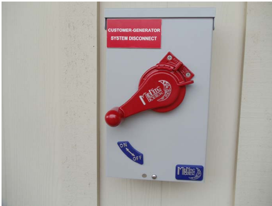
Figure 6 The cover/handle assembly installed with disconnect plaque reinstalled onto the new MidNite disconnect.
