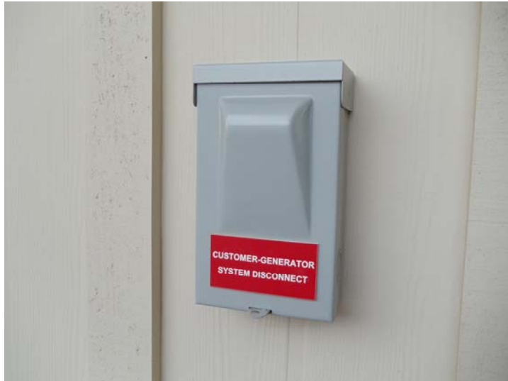
Figure 1 Square D pull switch. Works fine, just not what the customer wanted.
