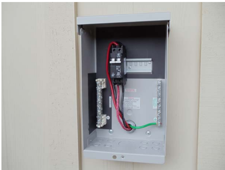
Figure 4 The Midnite MNPV6 Disco enclosure installed in place of the pull switch. A 2 pole 30 amp AC breaker is installed in the enclosure (MNEAC30-2P). The Neutral busbar is not used in this installation.
