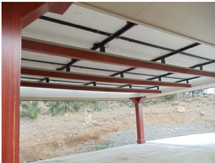
Figure 8 Underside of the 5000 watt array. The customer wished for a carport style array where the solar panels do not show. This reduces output and requires additional module cleaning.
