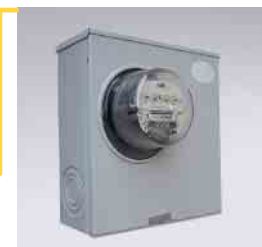
Electric Meter Measures incoming and outgoing electricity. Spins backwards when house PV system feeds power to grid.*
